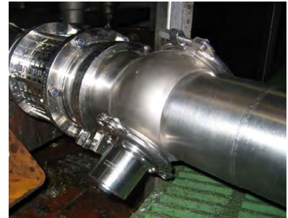
Sensor installed in pipe
