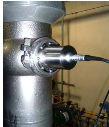
VS-1000C in-line installation at Brewery
